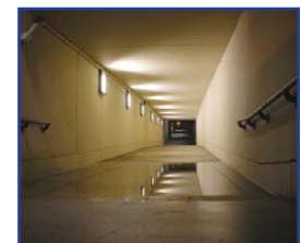
LEDtronics SLL003PC shoebox luminaires light up the pedestrian tunnel at Bolling Air Force Base in Washington, D.C.
